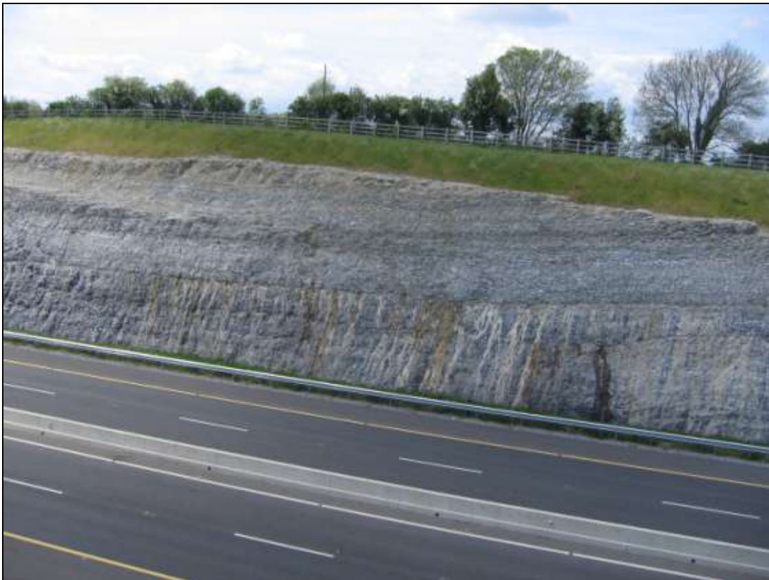
A view of the west side of the cutting clearly showing the changes in bedding half way up the face and the lime stains of water flows from the bedding plane of the junction.
